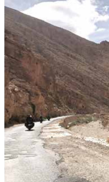
Not all the roads in Morocco are great. Many were, but some had eroded to the point where only part of the metalled road surface remained.
